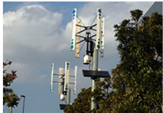
Hybrid streetlights installed at our Metropolitan Area Integrated Distribution Center (IDC)
