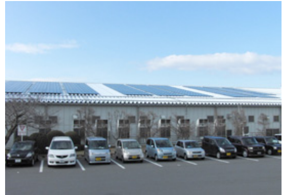
Solar panels installed at Shiga factory
