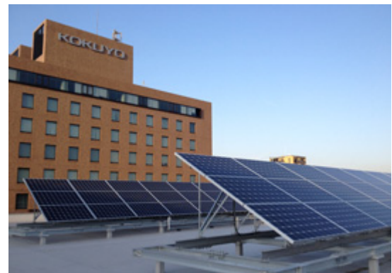
Solar panels installed at the new wing of our Osaka office
